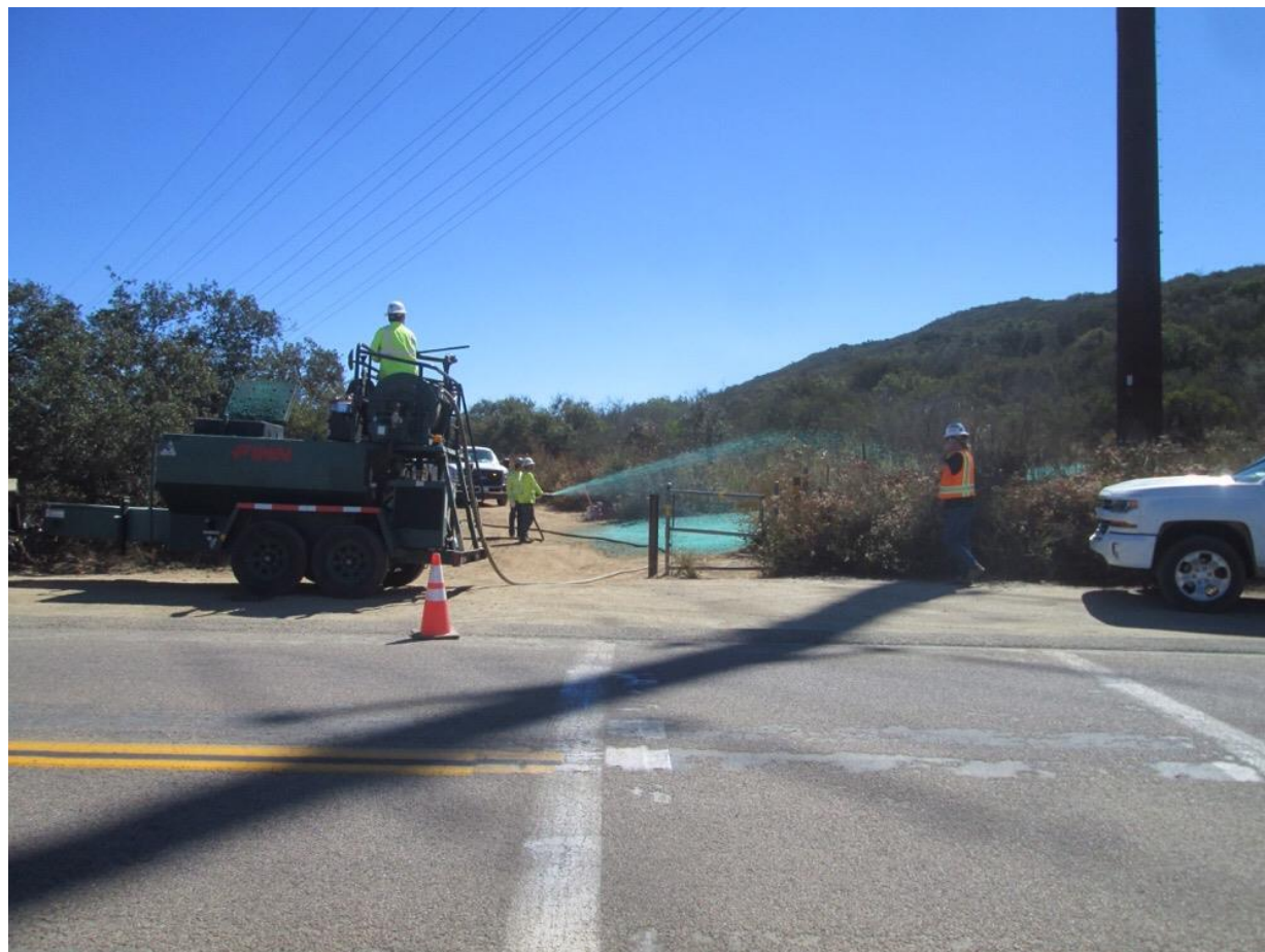
Photo 3: Hydro-mulch application at Z272860 (TL 625B) was observed in accordance with the Habitat Restoration Plan and project SWPPP. A biological monitor was present in accordance with MM BIO-3 and MM BIO-22.
