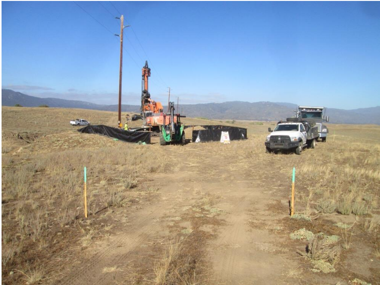
Photo 2: During pole hole drilling at Pole Z118216 (TL 682), the access road limits were clearly staked to prevent potential impacts to SKR in accordance with MM BIO-31.
