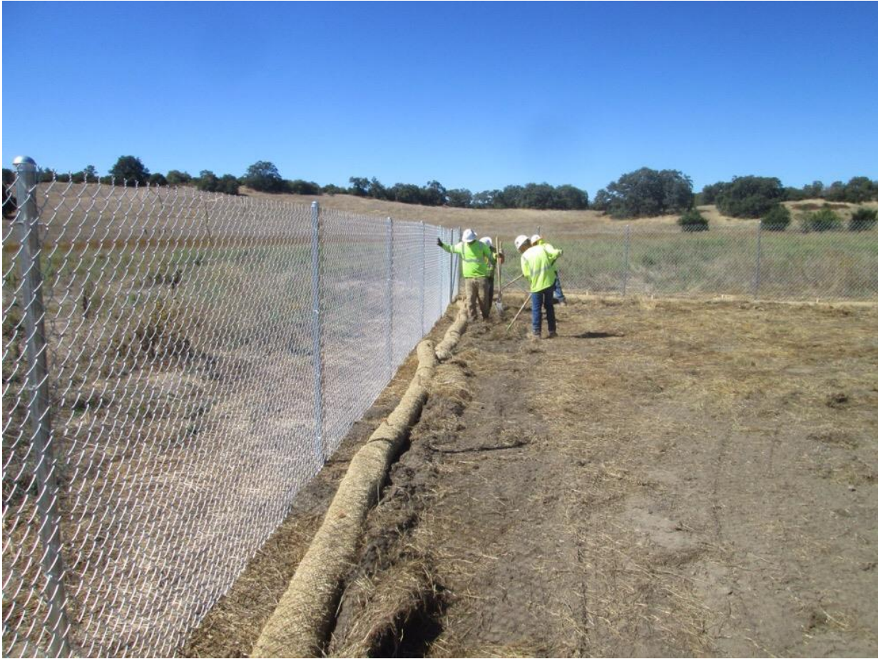
Photo 6: Crews installed perimeter fiber rolls at the Love Valley Staging Yard in accordance with the SWPPP and Erosion Control Plan.
