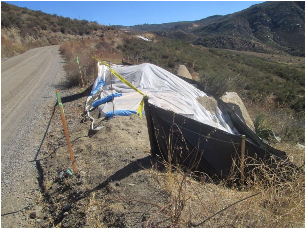
Photo 1: A completed pole hole was observed at P172688. The hole was covered to prevent wildlife entrapment in accordance with MM BIO-23 and the excavated spoil pile was covered with visqueen and surrounded by silt fence to prevent erosion in accordance with the project SWPPP (C 78).
